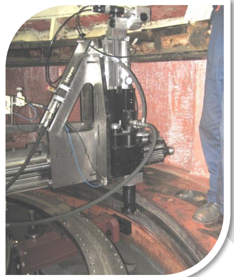
The purpose built assembly designed to accommodate a milling head and 200mm stroke.
