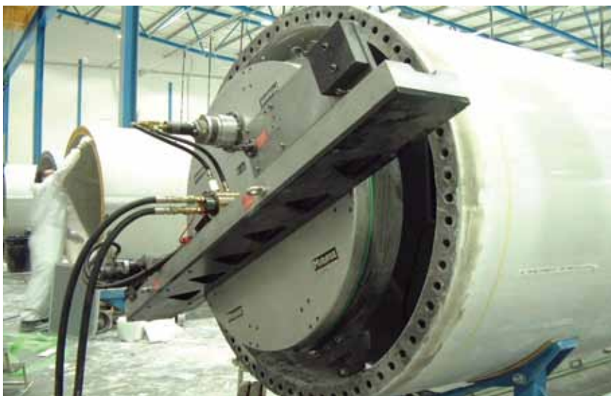
Left: the WP2500 system machining a 43m blade end in the UK.
